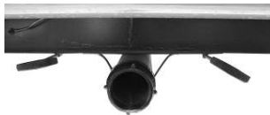
Black/Grey Tank Drain and Valves
